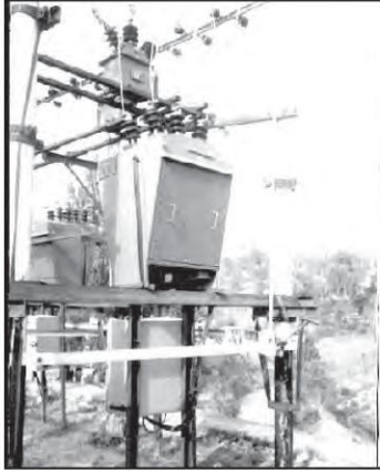
Fig. 6.1: An auto-recloser breaker and control unit at HPSEB in Himachal Pradesh
