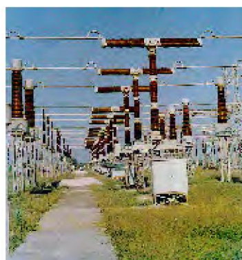
Live tank breaker (Courtesy BHEL)
